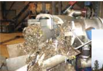
▲ Biogas station in Norway (photo: Bellona)
