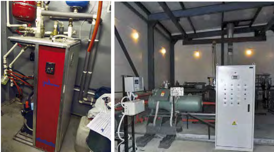
Left: Geothermal energy installation in Murmansk (Foto: Bellona)
