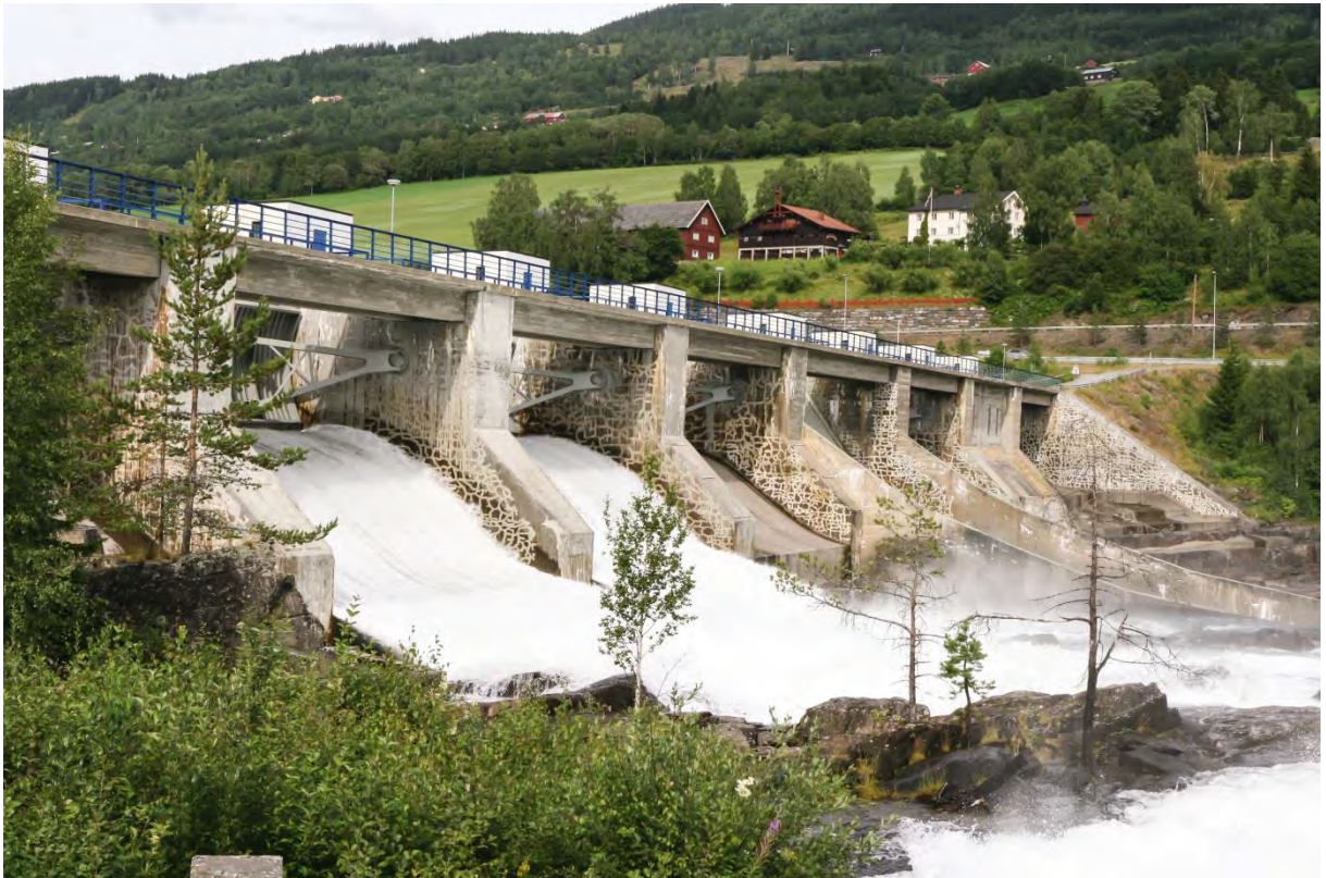
Hydro Power Station. Photo: Thinkstock
