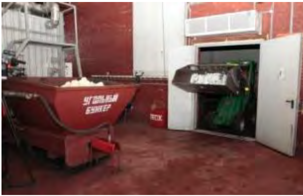
Wood pellets instead of coal (Foto: Bellona)
