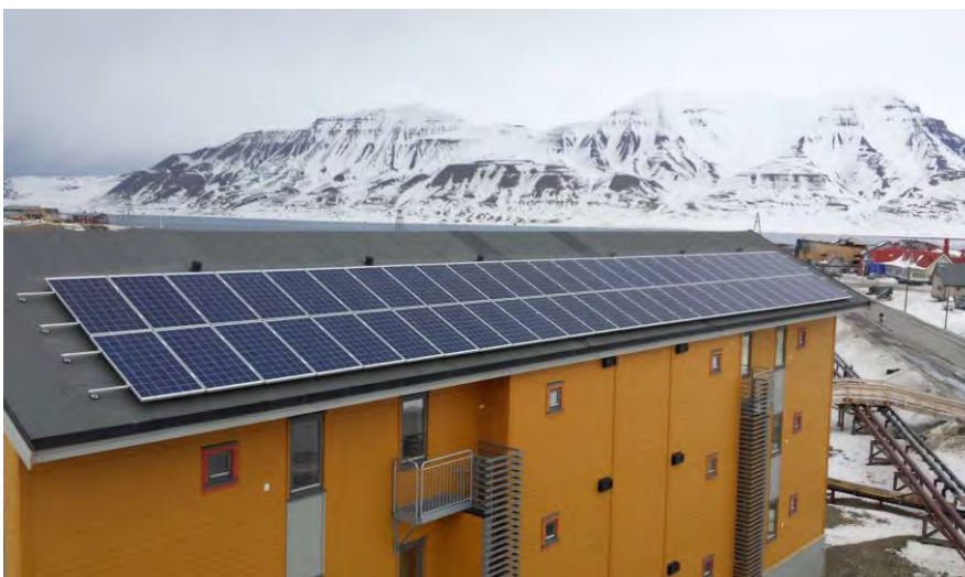
Solar panels installed in Longyearbyen, Spitzbergen Photo: Solbes (2015)
